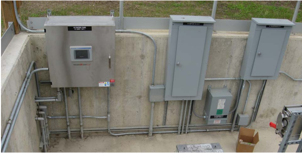
Trojan Technologies 3000 Plus Controls Center
