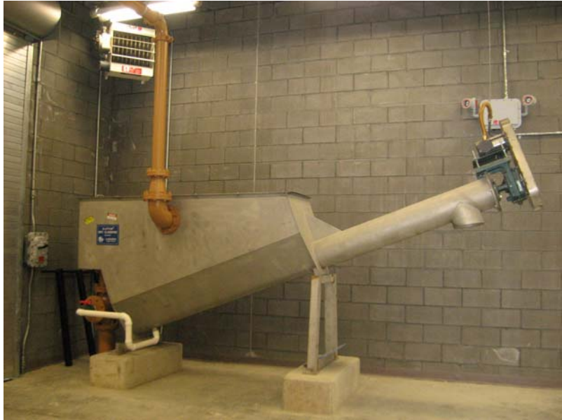
Lakeside Equipment Type L Grit Classifier
